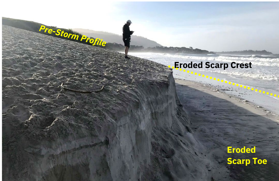
Figure 8. Dune scarp at Del Mar Sand Ramp. The yellow hatched line represents the previous summer’s beach profile. Dune scarping can have a significant impact on beach access. Source: City of Carmel, January 2023
