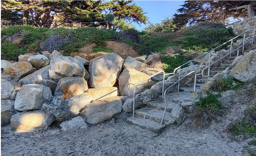
Figure 21. Stairway at Santa Lucia Avenue. Note damage to the railing from past storms.
