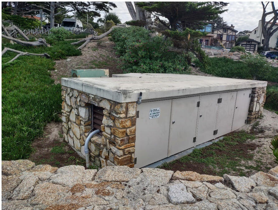
Figure 24. Wastewater lift station near 8 th Avenue.
