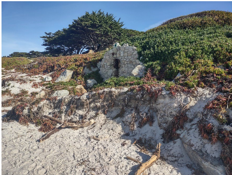
Figure 23. Stormwater drain near 8th Avenue fronted by an eroded scarp following winter storms in 2023. Note the riprap boulder on the bottom right.
