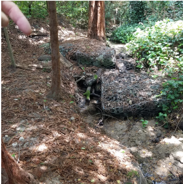
Photo 6: Looking Upstream at a failing gabion weir with a spillway that is undersized for even moderate storm events.
