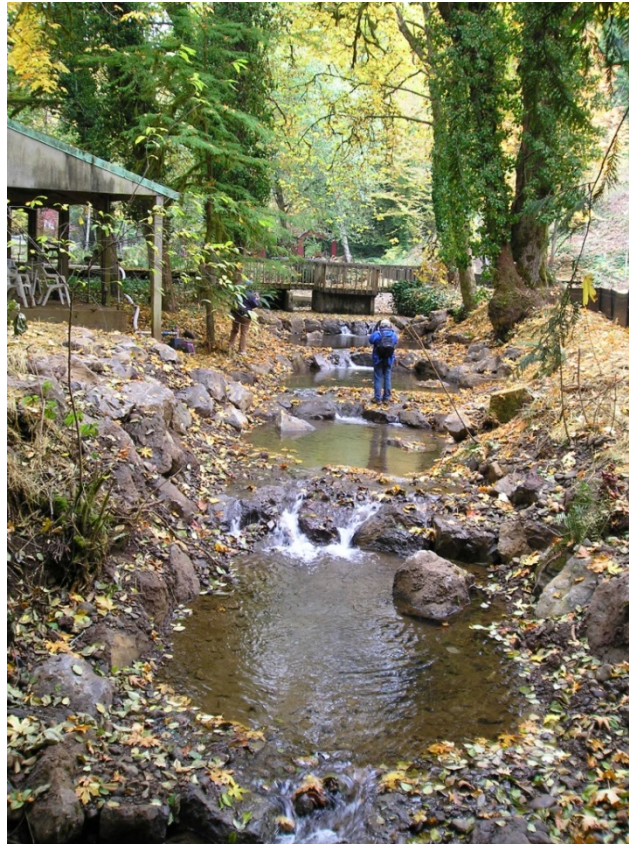
Photo 4: Example of boulder weirs used to raise a channel profile to support an existing bridge (Murtaugh Creek, OR)
