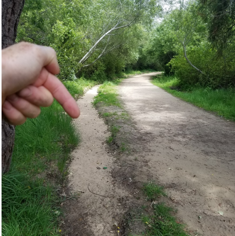
Photo 1: Sedimentation of ditch near station 8+00
