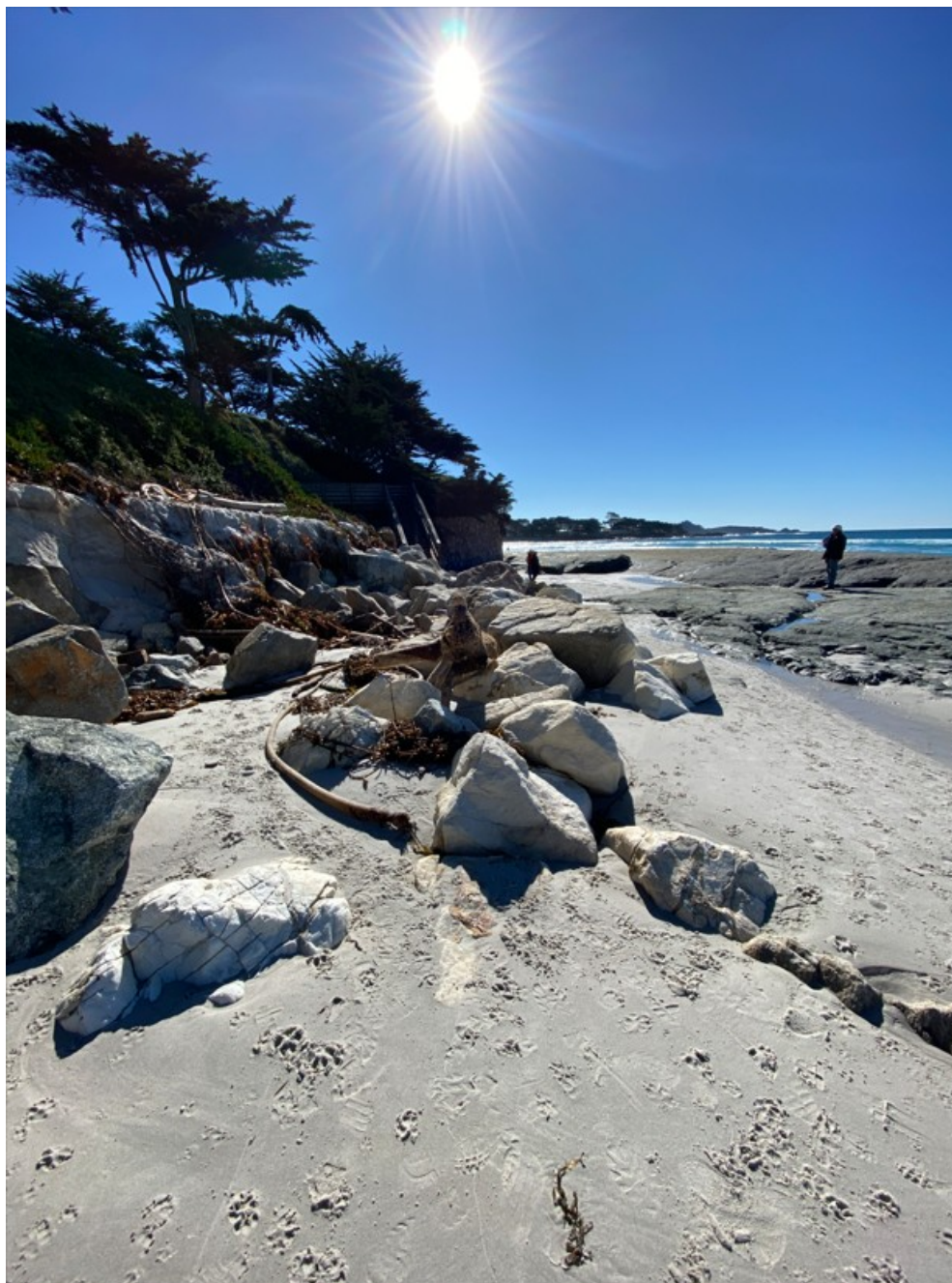
Photograph 76: Showing Collapsed Southern End of Revetment R5 on January 30, 2023
