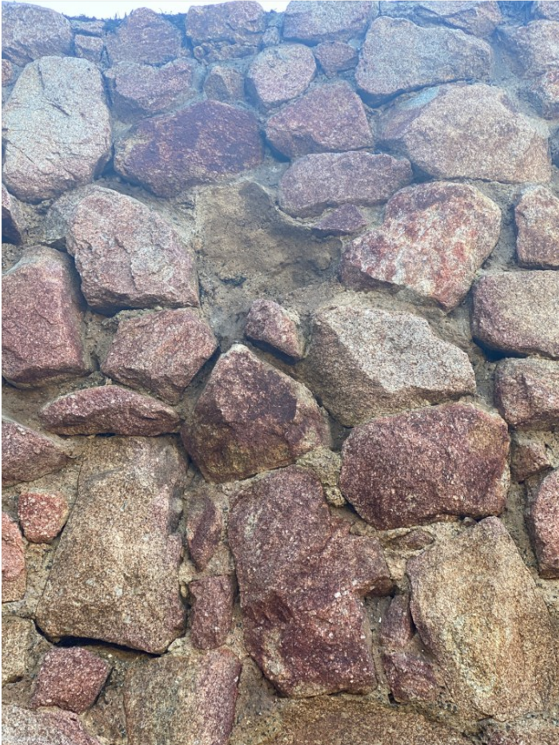
Photograph 26: Seawall S3 Showing Missing Rock on December 22, 2022
