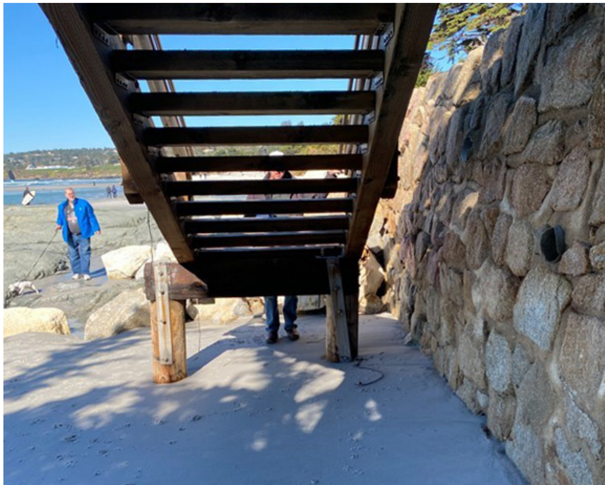
Photograph 74: Stairway ST7 on January 30, 2023 Showing Undermining
