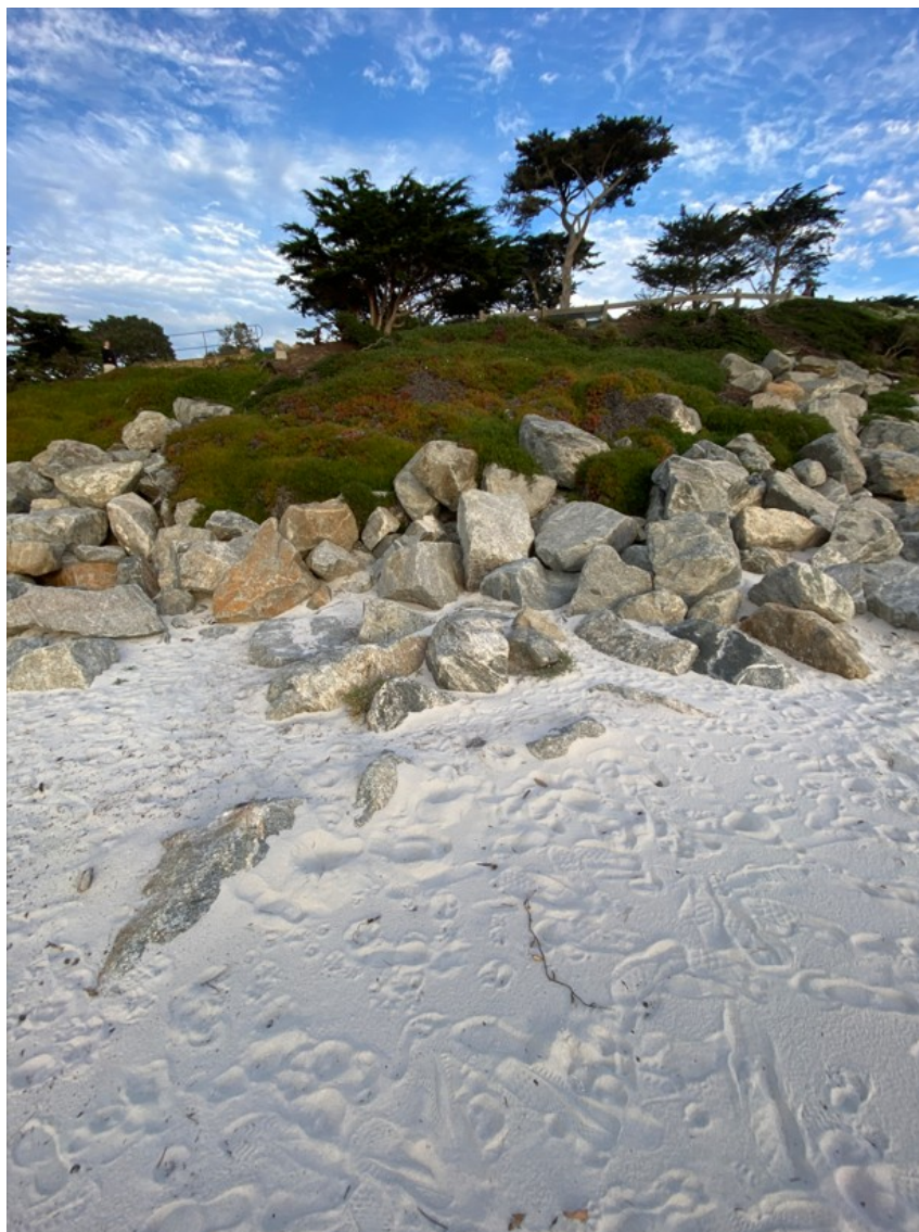
Photograph 48: Revetment R3 Showing Area of Rip-rap on December 22, 2022 Where the Public Could Benefit from Quarystone Re-stacking
