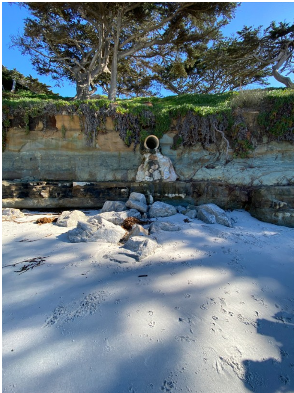
Photograph 44: Storm Drain Outfall with Minor Armoring Between ST4 and R3 on January 30, 2023
