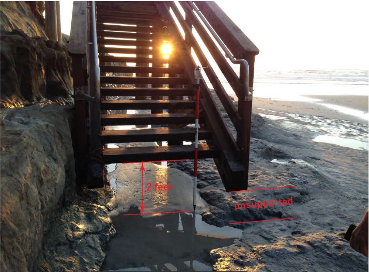
Photograph 39: Undermined Stairway ST4 in February 2016 (Easton Geology)
