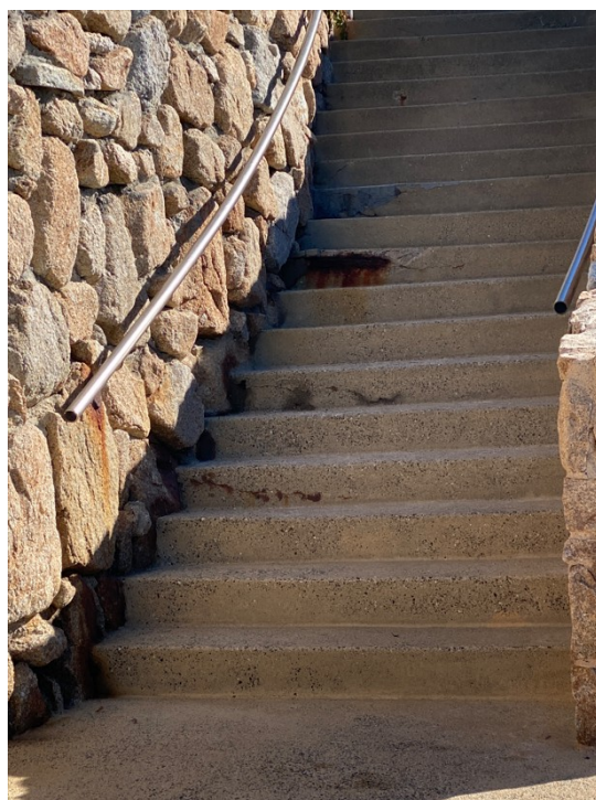
Photograph 67: Stairway ST6 with Tread Deterioration on January 30, 2023
