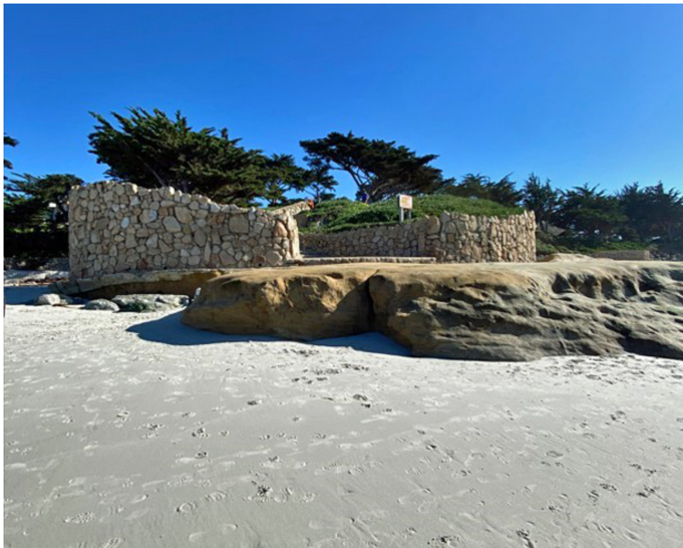
Photograph 28: Showing Public Access Stairway ST3 with Seawall S3 on Both Sides On January 30, 2023
